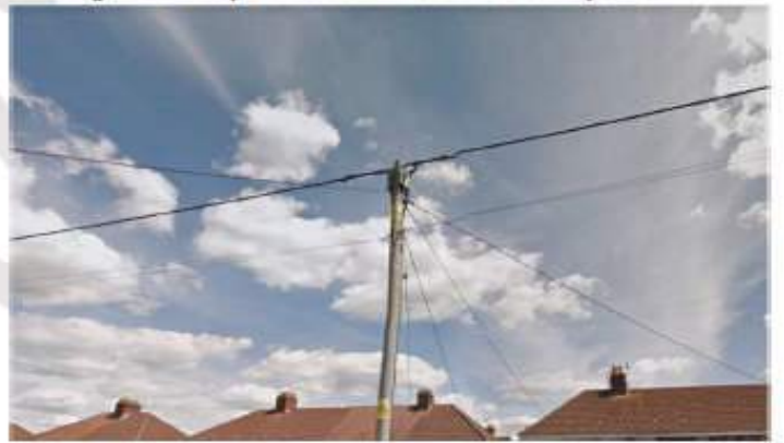
LV electricity pole with both electricity wires and telegraph wires coming off it. The electricity wire is at the very top of the pole and the thinner telegraph wires are located lower down on the pole. They also spread out from the pole whereas the electricity wire forms a straight line.
